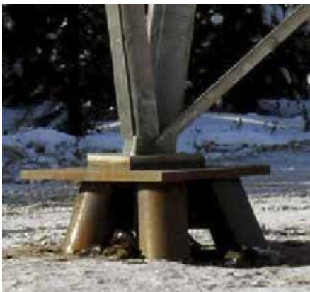
Helical Pier Foundation. Materials: Prefabricated Steel Piers and Base Plates Equipment: Modified Excavator, Small Crane
